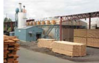
A vertical heater extending through the roof of the building located next to the kiln has two helical coils arranged so that burner gasses make three passes over their surfaces before entering the exhaust stack.
