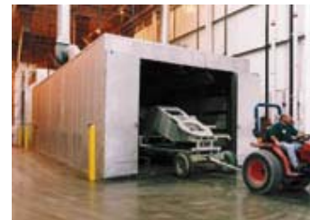
A 6,000 lb hydraulic crane upper frame is removed from the catalytic infrared curing oven for cool down.
