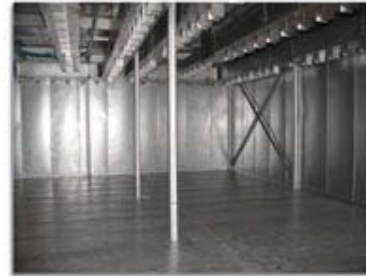
Figure 1. The oven should have a clean, smooth insulated floor. Locating the hot air supply ductwork in the ceiling eliminates the problem of parts falling off and damaging the ductwork.
