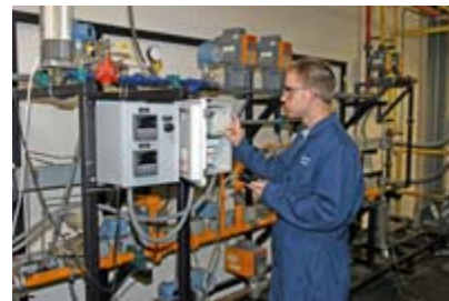
Today, burner manufacturers are integrating intelligent controls on burners to monitor air/fuel ratio and provide automatic adjustment.
